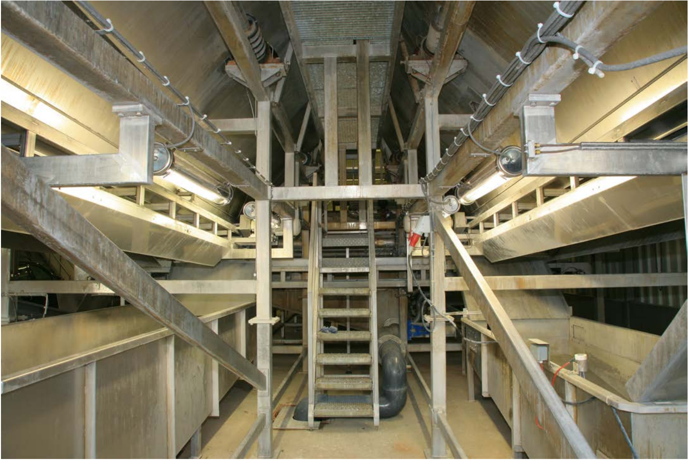
Wastewater treatment plant, HAK, Netherlands
