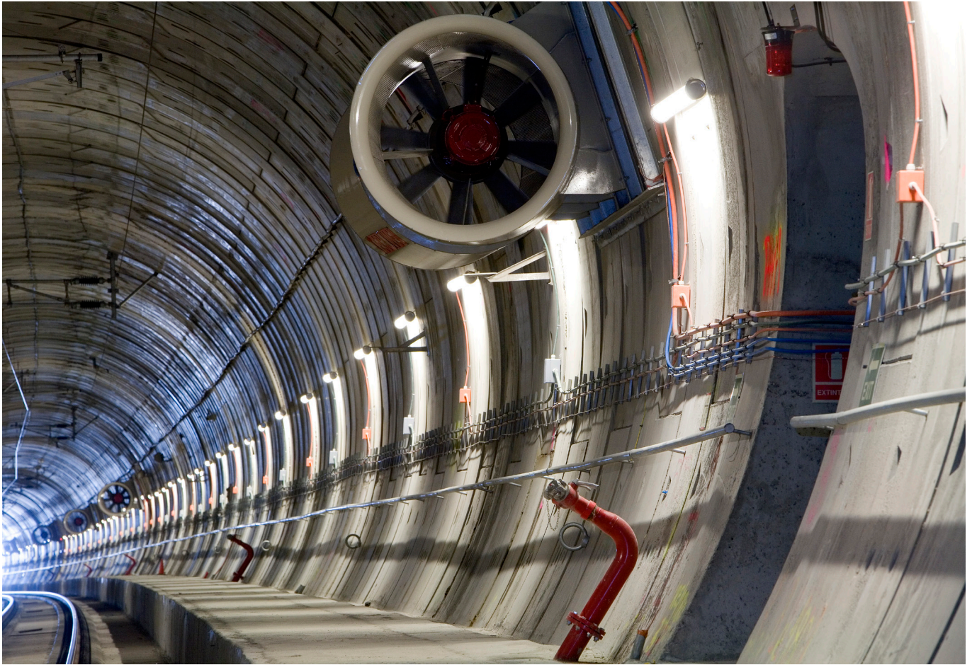
Perthus LGV tunnel between France and Spain.
