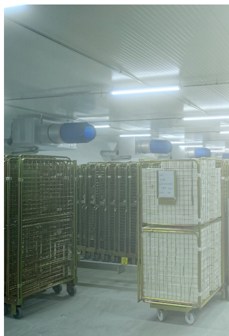
Cold room, France
