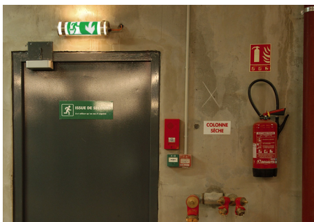
Emergency lighting - Coulomb BAES
