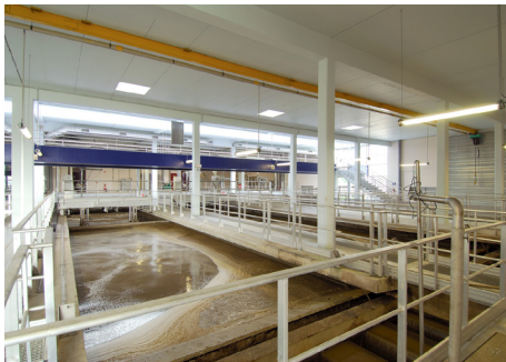
Water treatment facility, France
