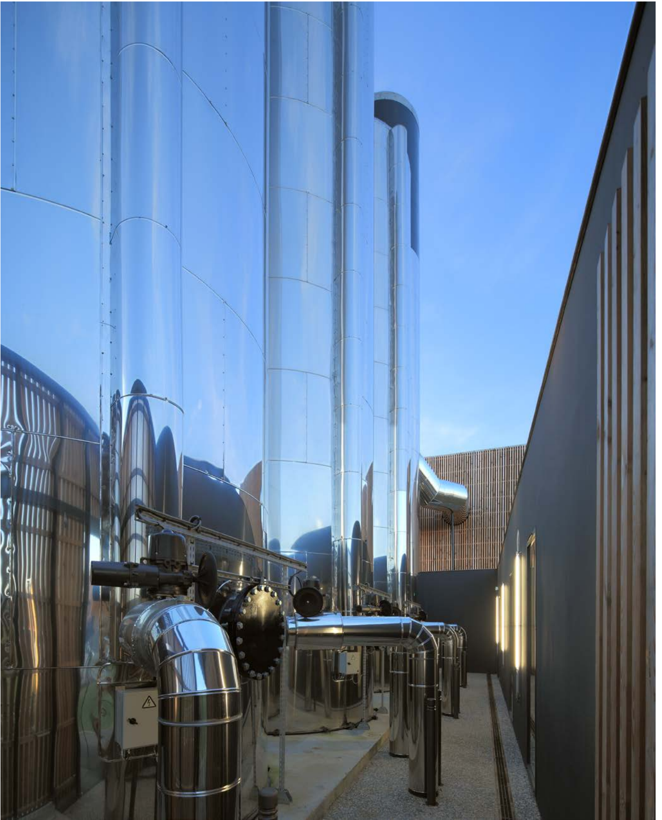
Boiler room, Dalkia, La Rochelle, France.
