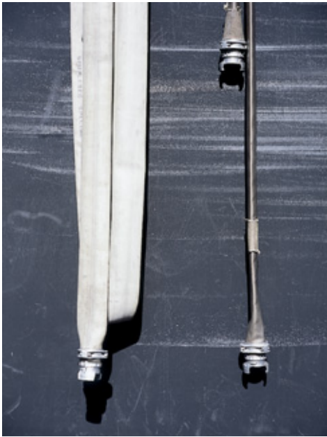
Fire hoses hanging against the painted concrete wall of the training tower.
